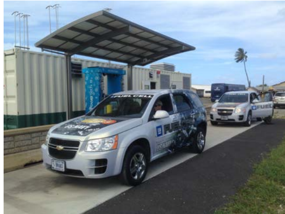
MCBH Hydrogen Station
