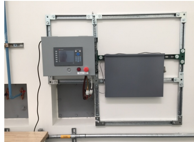
Relief valve programmable logic controller (PLC) control box
