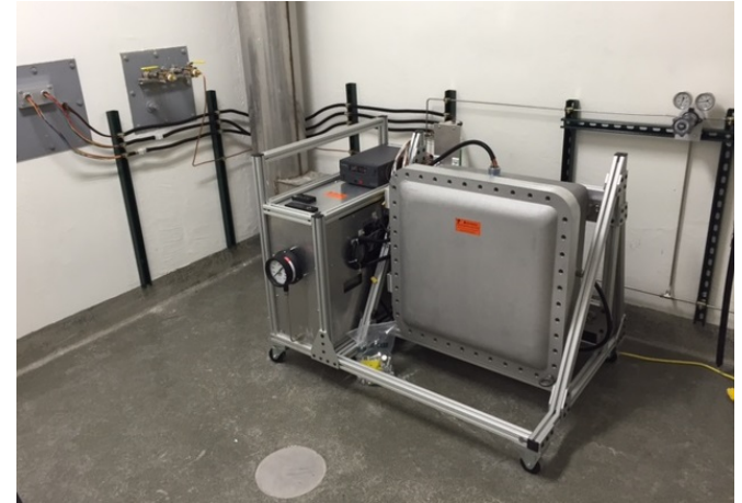
Relief valve apparatus installed in ESIF high pressure test bay
