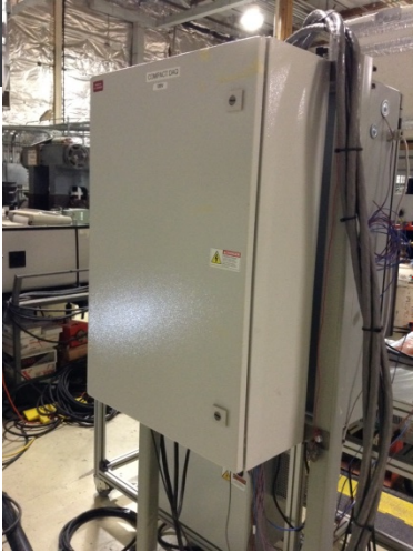
Data acquisition panels
