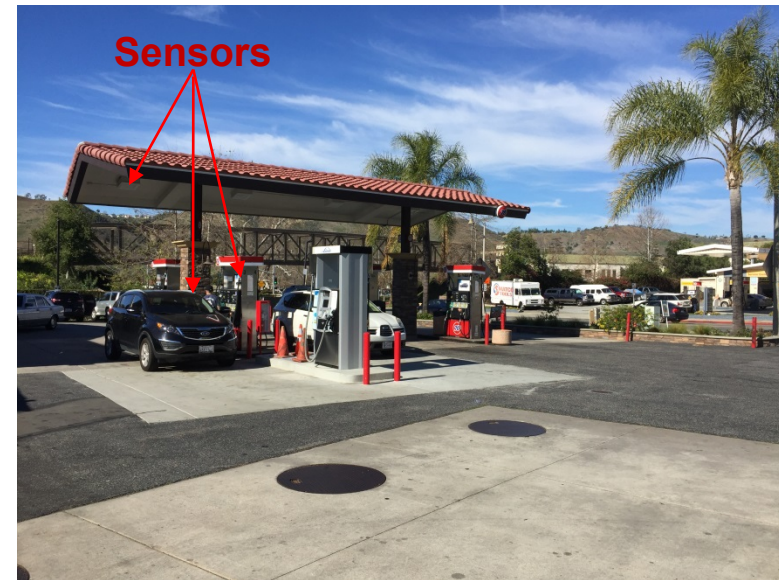
Hydrogen sensors in and around a hydrogen dispenser and FCEV
