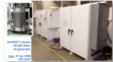
Figure 1. SunHydro #1 Compression, Storage, Dispensing Containerized System
