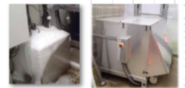
CO2 Heat Exchanger R. 20-ton cylinder behind 2 hr Storage
