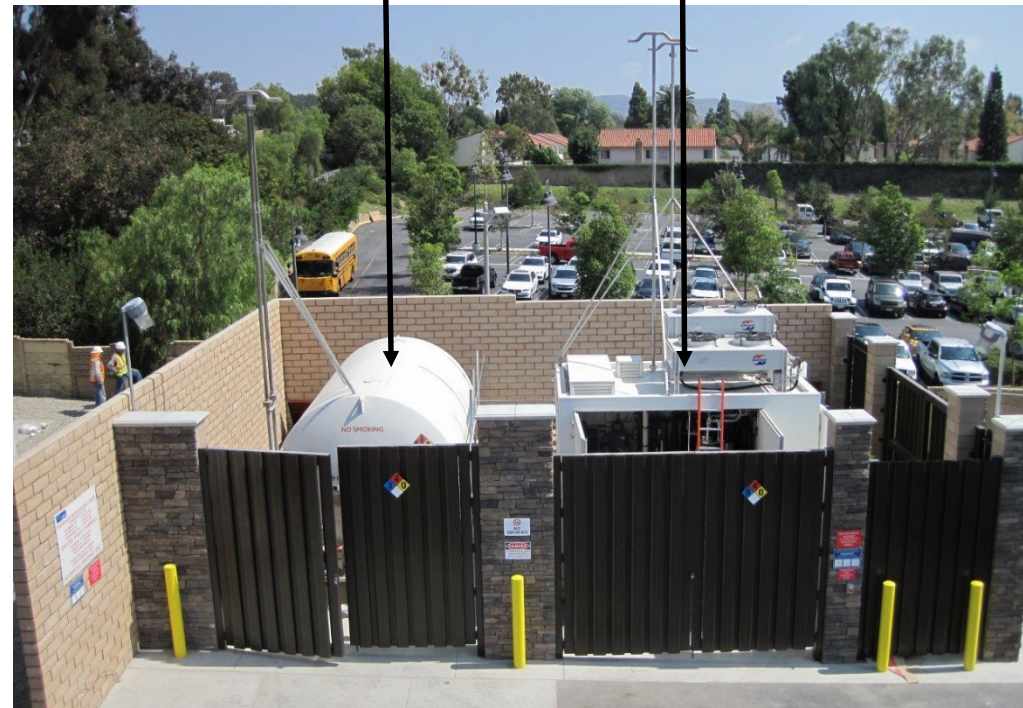
LH 2 Storage GH 2 Compressor Linde Storage and Compression Equipment at San Juan Capistrano
