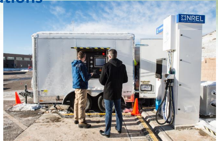
NREL's Hydrogen Infrastructure Testing and Research Facility
