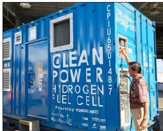
Maritime fuel cell 100 kW generator
