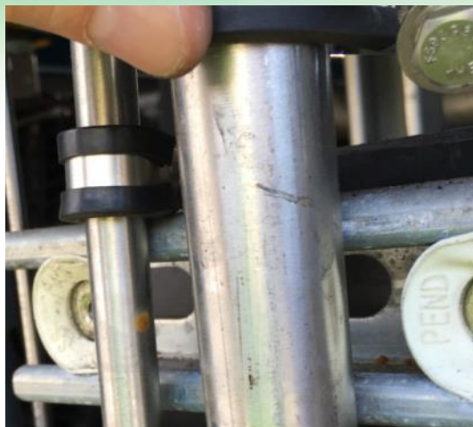
Stainless steel piping under rubber clamp
