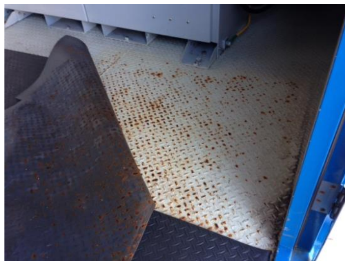
Painted carbon steel floor with trapped moisture
