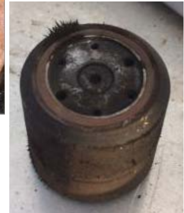
Failed check valve
