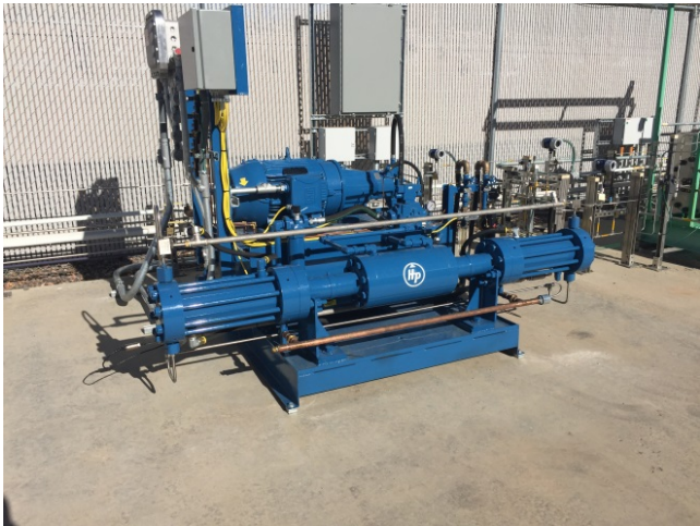
Hydro Pac – Upgraded high pressure compression capabilities to 18 kg/hr
