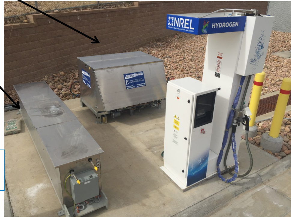
2017 - Dispenser with new chiller and triple block heat exchanger
