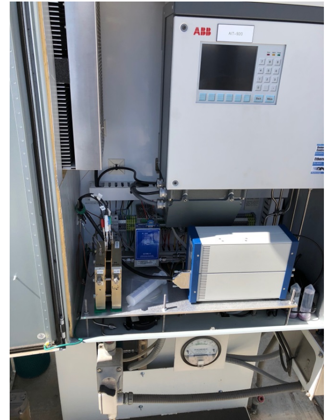
LANL HCD installed at H2F, Burbank, CA
