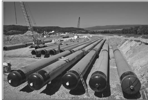
NG Pipe Storage, Erdgas, Switzerland
