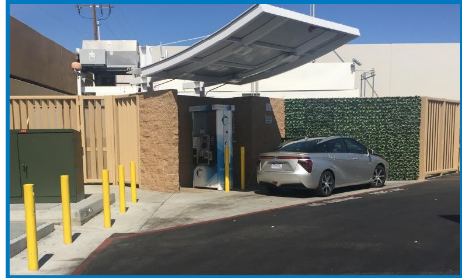
Air Liquide, Anaheim, CA. Photo: NREL
