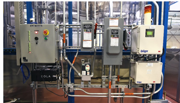
Gas alarm and Interlock System
