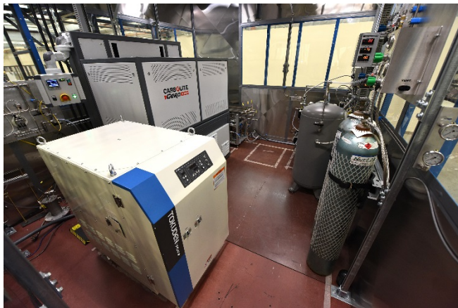
Enclosure Interior View
