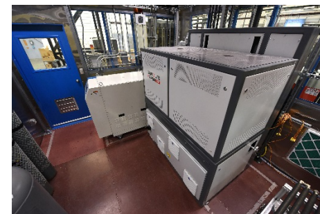
25 kW HTE test station hot zone and steam generator
