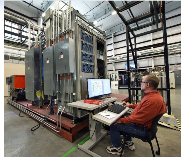
25 kW HTE Test Facility Control Station
