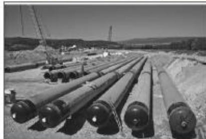
NG Pipe Storage, Erdgas, Switzerland
