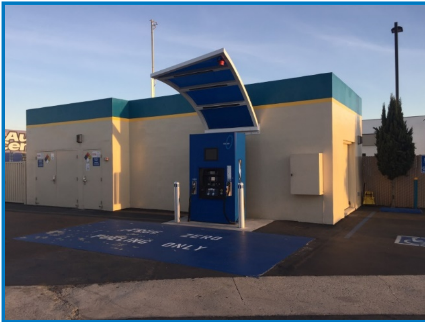
FirstElement Fuel, Costa Mesa, CA. Photo: NREL
