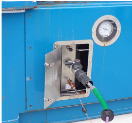
Successful H 2 connection, grounding truck to unit.
