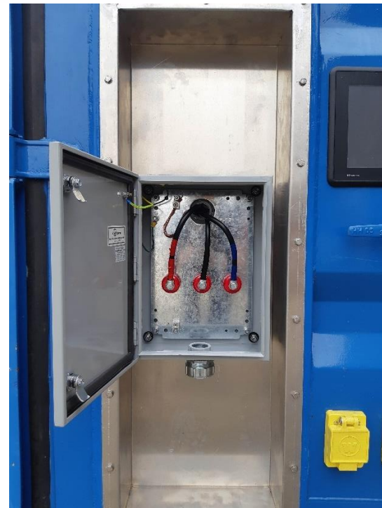
New recessed connector panel/box mounted on the MarFC unit to SIO specifications.
