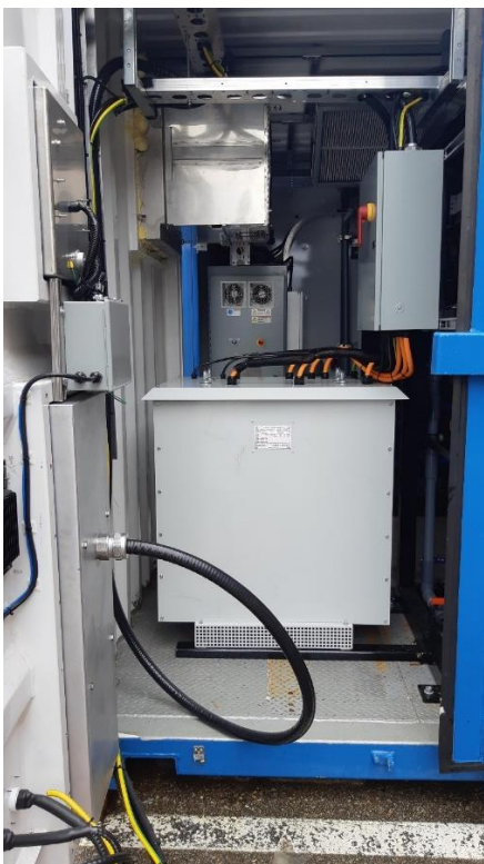
New 480VAC transformer installed
