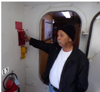
Powering fire pump systems
