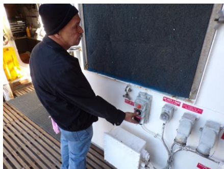
Powering Deck Pump.
