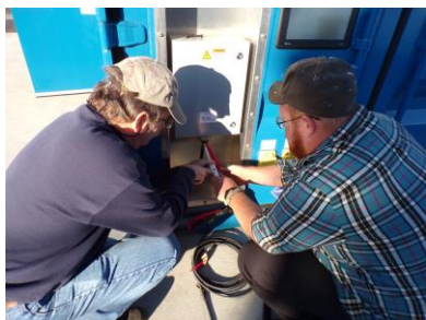
Connecting vessel cable to MarFC.
