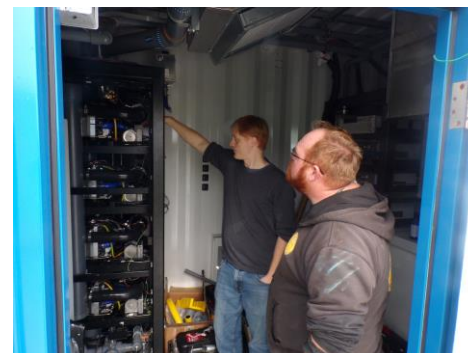
...and then of the fuel cell rack and power electronics
