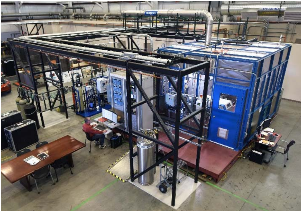
25 kW HTE Facility
