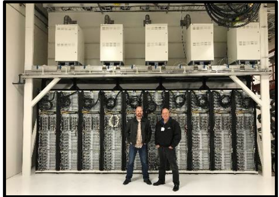
Datacenter at Microsoft Advanced Energy Lab
