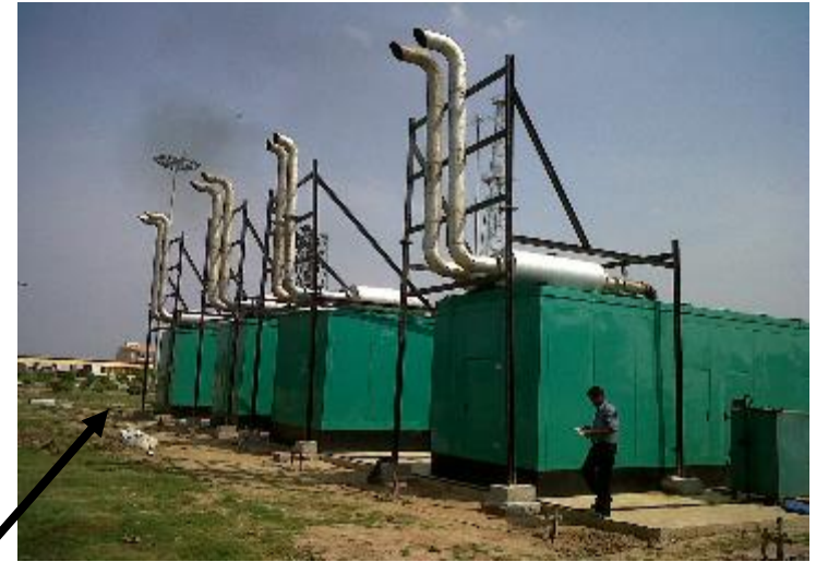
Diesel Generators in India
