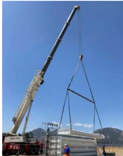
ARIES H 2 System at NREL Flatirons Campus
