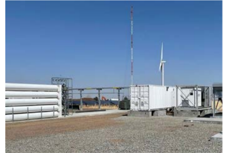
ARIES H 2 System at NREL Flatirons Campus
