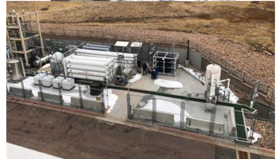
NREL's HD Hydrogen Infrastructure Testing and Research Facility
