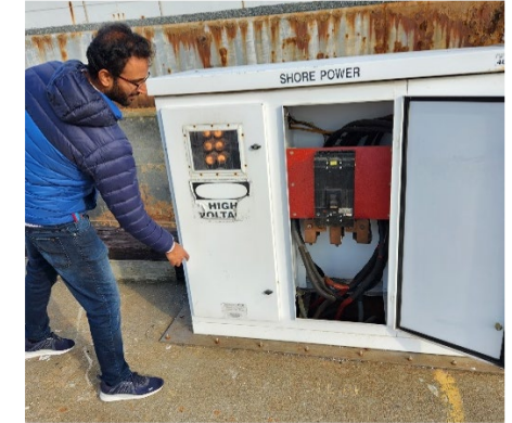
Raman Singh inspects a 480VAC shore power box on Wharf 3.
