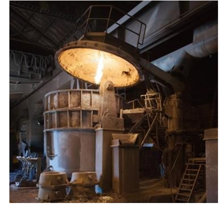
Steel Mill Ladle Heater
