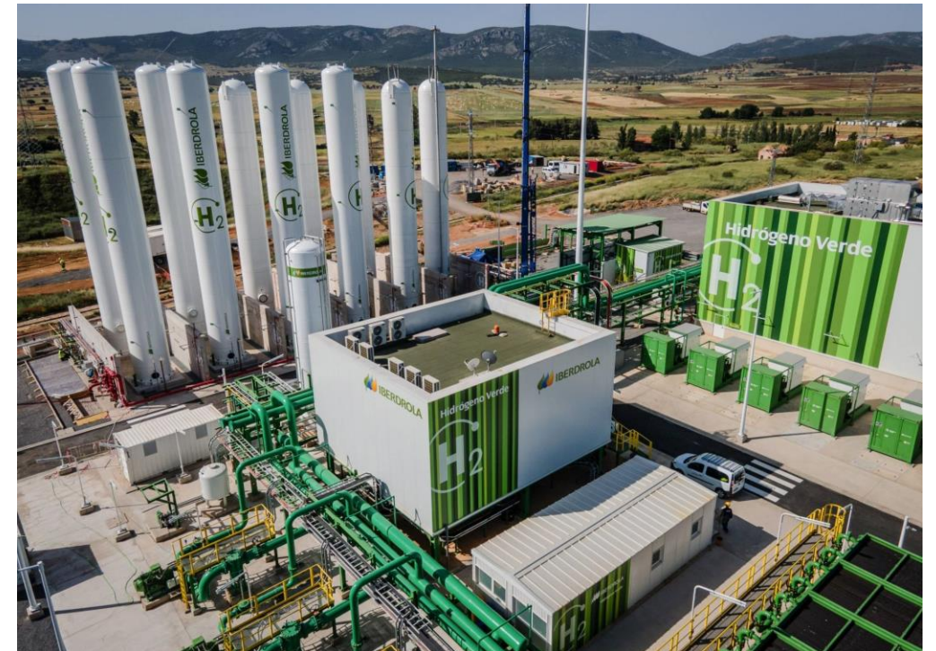
Multi-MW PEM installation
