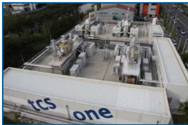
Four 2.8 MW FuelCell Energy power plants providing clean power to the South Korean electric grid
