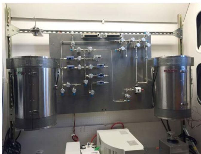
FIGURE 3. Photograph of the existing state of the flowing particle reactor test system
