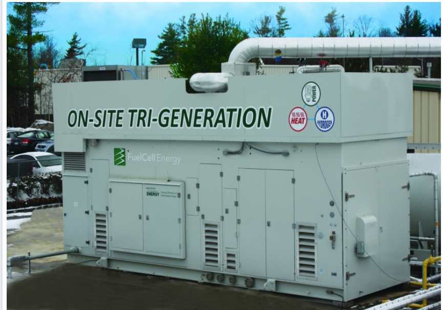
The high efficiency packaged CHHP system in operation at FuelCell Energy's manufacturing plant in CT .
