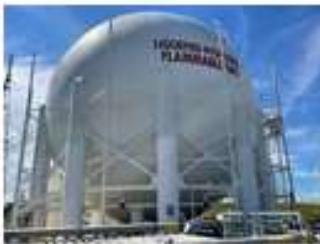
LH 2 storage tank 5,000 m 3
