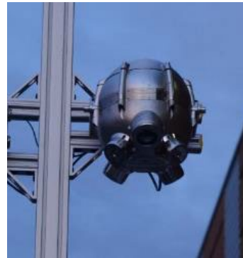
Commercial ultrasonic leak detector installed at NREL
